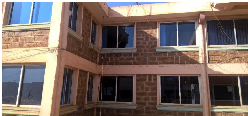
Figure 8.1: Busia Kenya: Spider Web of Electrical Cables on Building
